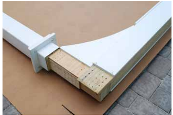
Align Post and Header Beam with Arch Brace tightly together from top to bottom.
