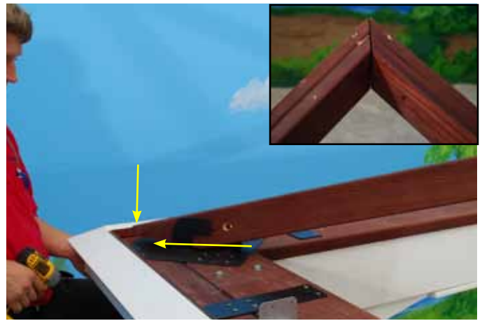
Slide Double Hip Rafter into Corner Plate and pressed snugly into corner.
