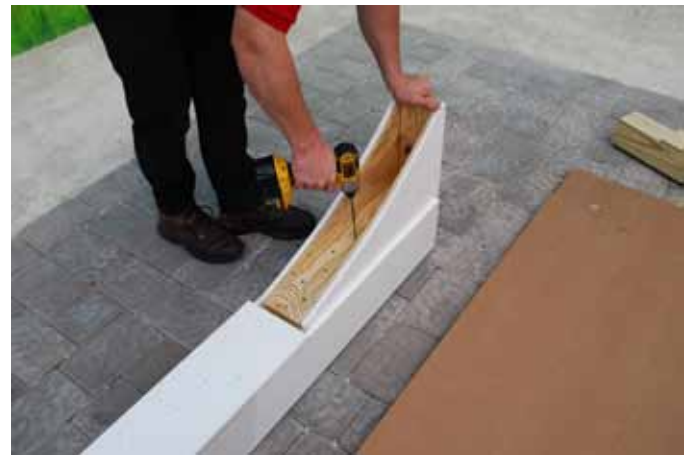
Attach Arch Brace to Header Beam using 3.1/2" Brown Screws through pre-drilled holes
