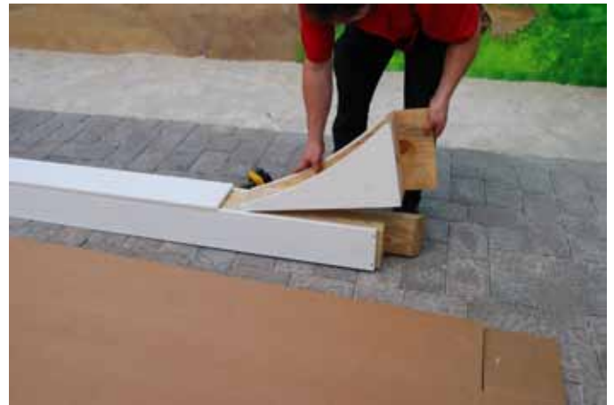
Install Arch Braces, There are left and right side arch braces. Place Correct one on each side as shown.
