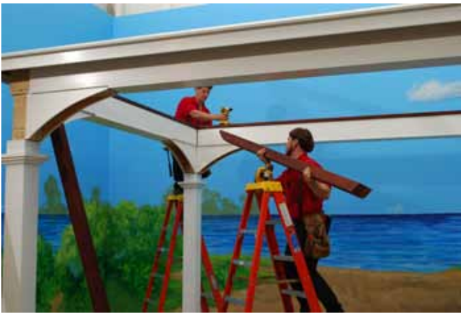
Install first Double Hip Rafter. There are 2 Left & 2 Right Rafters. Be sure to install them in proper corners.
