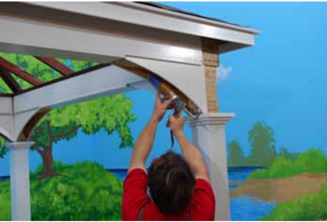
Apply Liquid Nails inside Arched Header on both sides where 2x4 Corner Brace will be fastened
