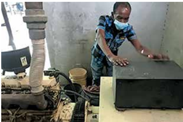
Noel in the maintenance room checks the generator
